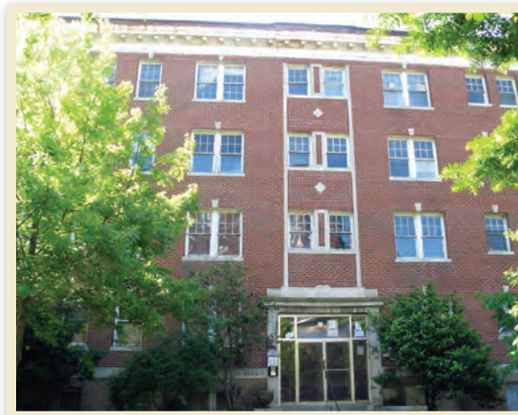
The St. Dennis Apartments is one of many applicants competing for federal weatherization funds in Washington, D.C.
